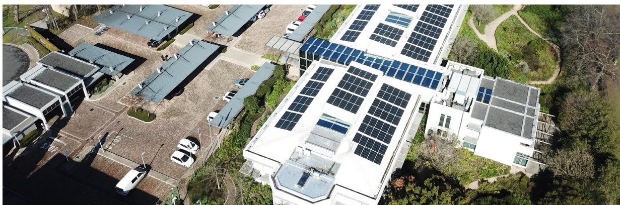
The rooftop photovoltaic system on top of Remgro's Millennia Park Building
